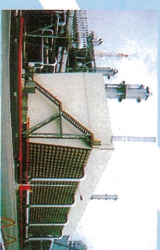
Crossflow type Cooling Tower for industrial process cooling
