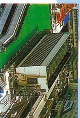
Crossflow type Cooling Tower for district cooling
